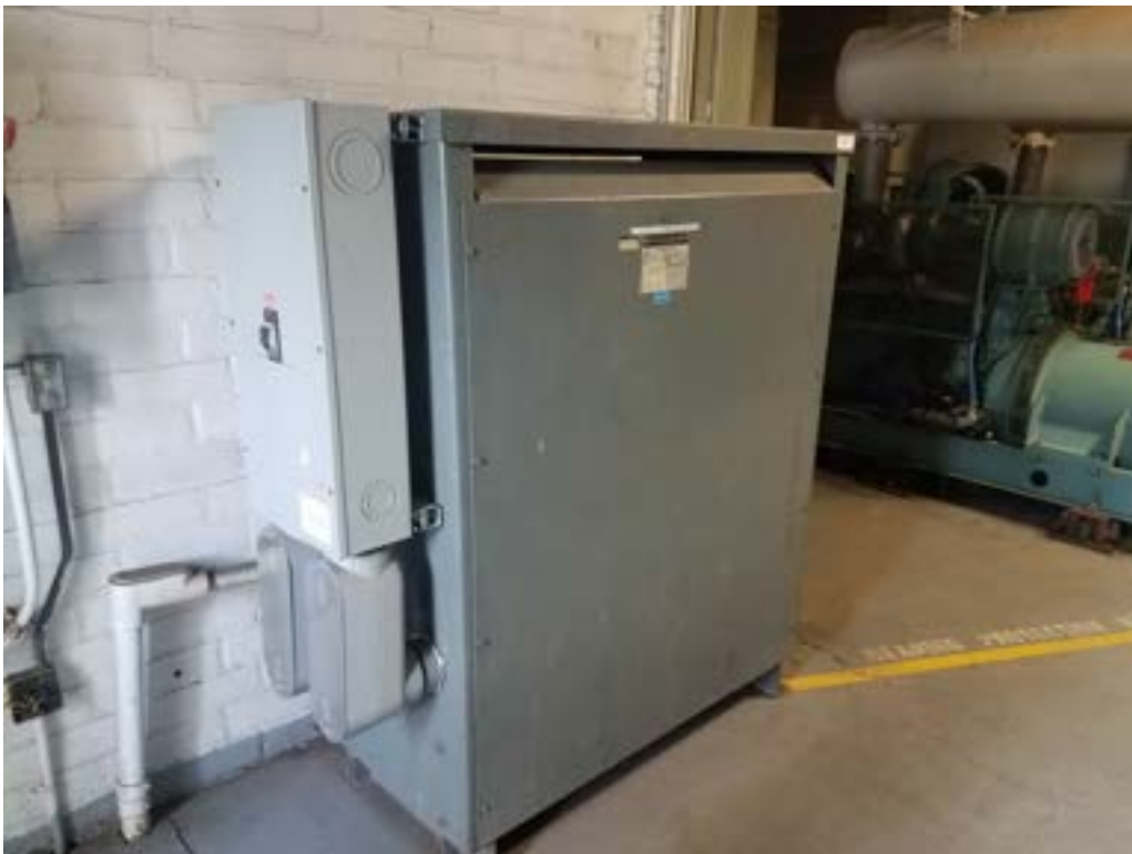
View of transformer in maintenance building.
