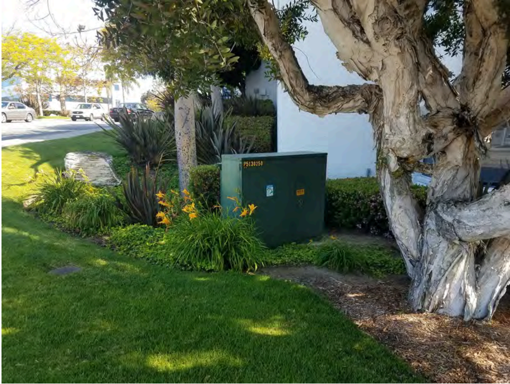
View of typical utility-owned pad-mounted transformer as seen on Parcel 1.
