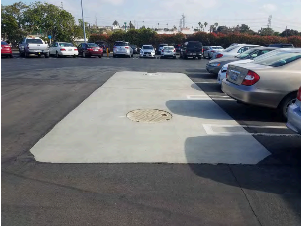
View of concrete patch and fill ports above the 10,000-gallon diesel fuel UST.
