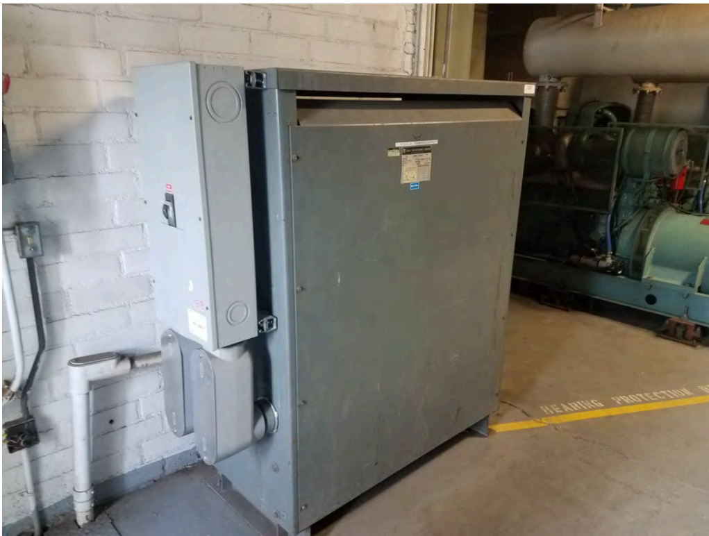
View of transformer in maintenance building.
